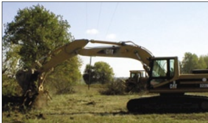
Mike and Jody Zwahlen dozing trees out of the line at Verl Shufelt's.
