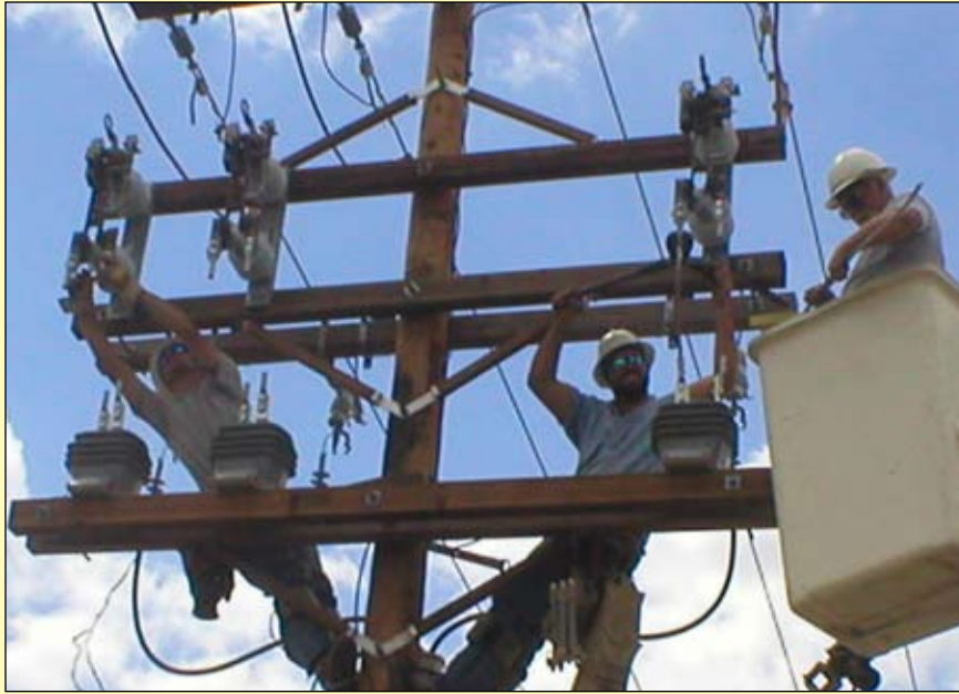
From left to right: Kyle Schaper, Journeyman Lineman; Tyler Kennett, fourth year Apprentice Lineman; and Tom Shelton, Crew Foreman, are shown installing three current transformers to improve the Altamont Metering point for TWACS. TWACS is an automatic meter reading system that will allow the office to retrieve readings and monitor members' usage.
