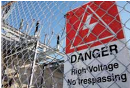
Never go into an electric substation for any reason. Electric substations contain high-voltage equipment, which can be deadly.
