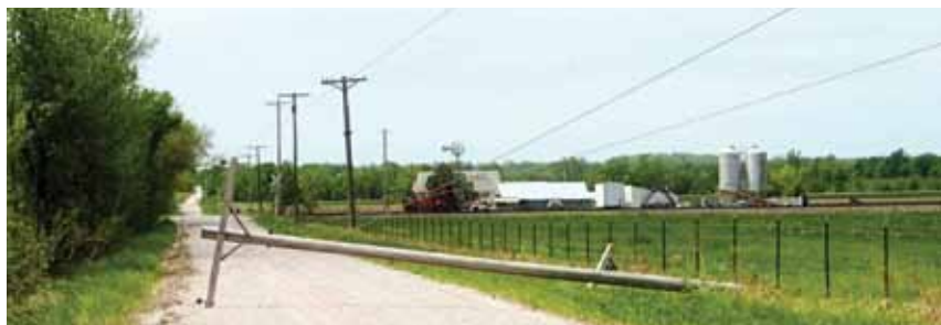
Many members were left without power after the windstorm due to fallen power lines.
