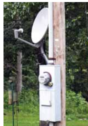
Satellite dishes and other unauthorized attachments must be removed to protect lineworkers.
